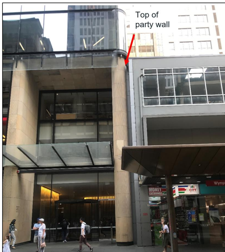
Figure 39: View of existing party wall from George Street, with top of party wall indicated
